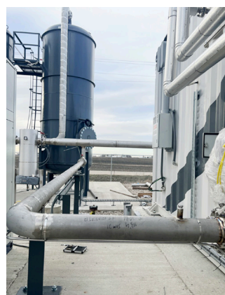
H 2 S AND STAINLESS-STEEL PIPE RUN
