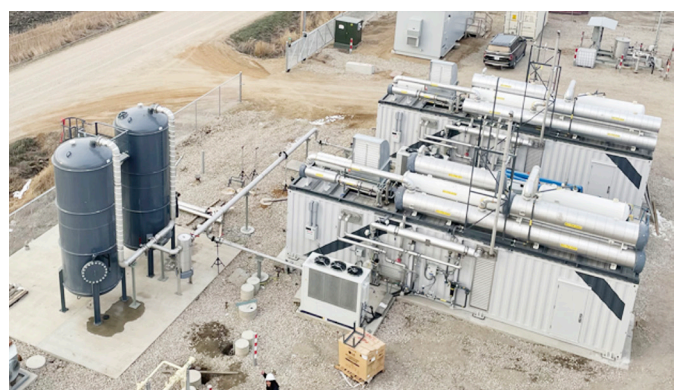
NEWLY INSTALLED BIOGAS TREATMENT PLANT
