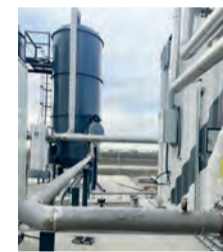
H 2 S and stainless-steel pipe run
