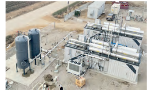
Newly installed biogas treatment plant
