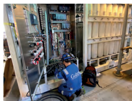
Goltens electrician installing a new Server Rack as per Safekick MPD design. This is the main control server for the MPD system
