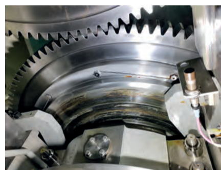
Damage to thrust collar during sea trial before repair
