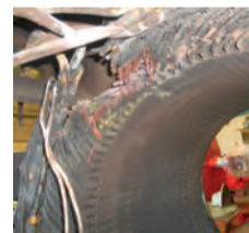
Damaged stator prior to rewinding
