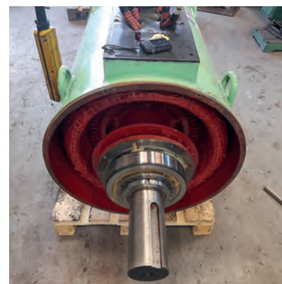
One of the many motors and pumps overhauled by Goltens Dubai
