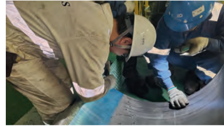
Scraping of intermediate shaft bearing
