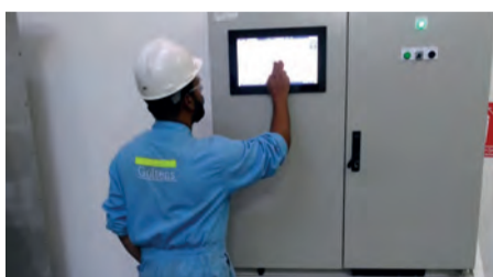
Goltens Energy Controls Solutions specialist configuring new load-shedding panel
