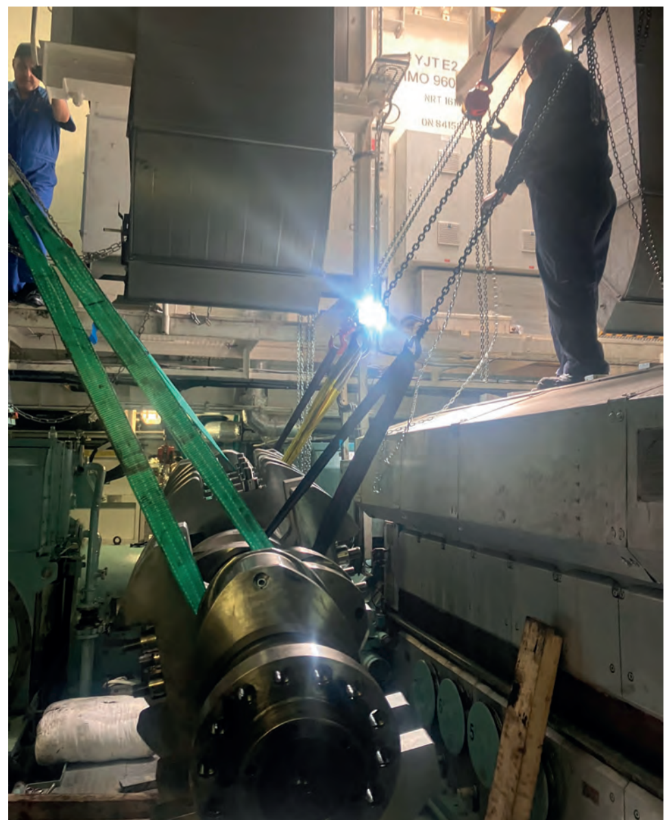
Rigging of the damaged crankshaft from the engine room to the upper deck
