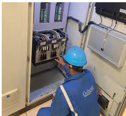
Goltens working on ITCC Cabinet with MicroNet Plus™
