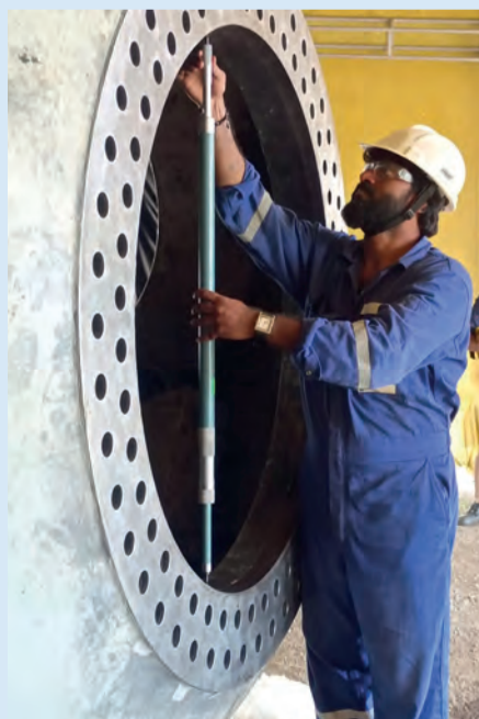
Goltens specialist performing calibration of the WTG hub inner diameter before machining
