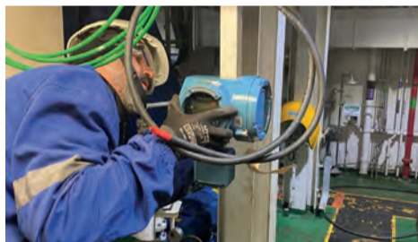
Electrical installation valve actuators
