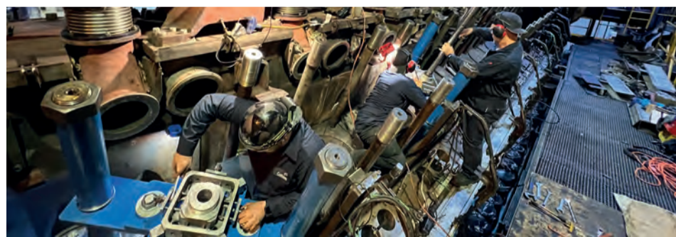
Installation of line boring equipment and dial indicators to check alignment of shaft to block and landing surfaces
