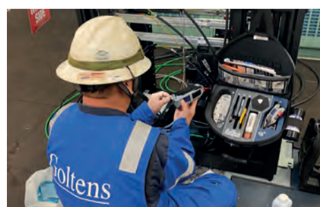
Goltens electrician integrating the new HPU unit for an MPD designed by Safekick allowing for communications between UPS, server rack, and HPU to properly function and communicate as per design
