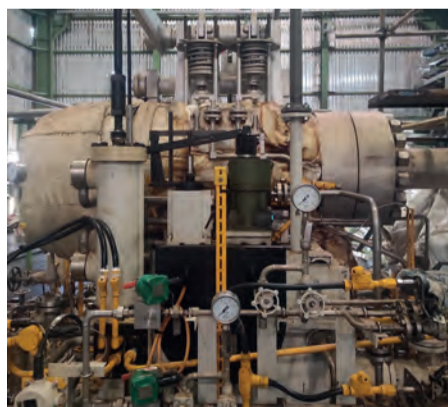
Dangote turbine with Woodward actuator
