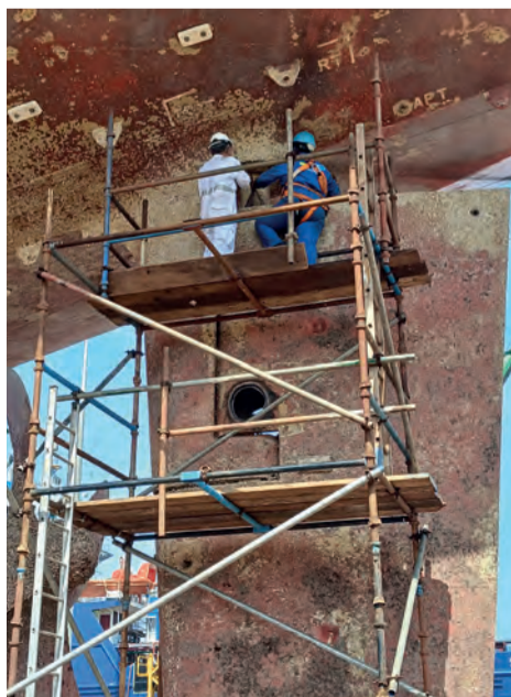
Rudder clearance check
