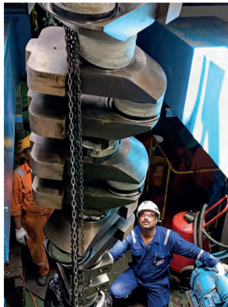
Rigging of damaged crankshaft from below decks for transport to Goltens Dubai
