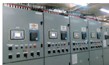
New Load Shedding Panel installed
